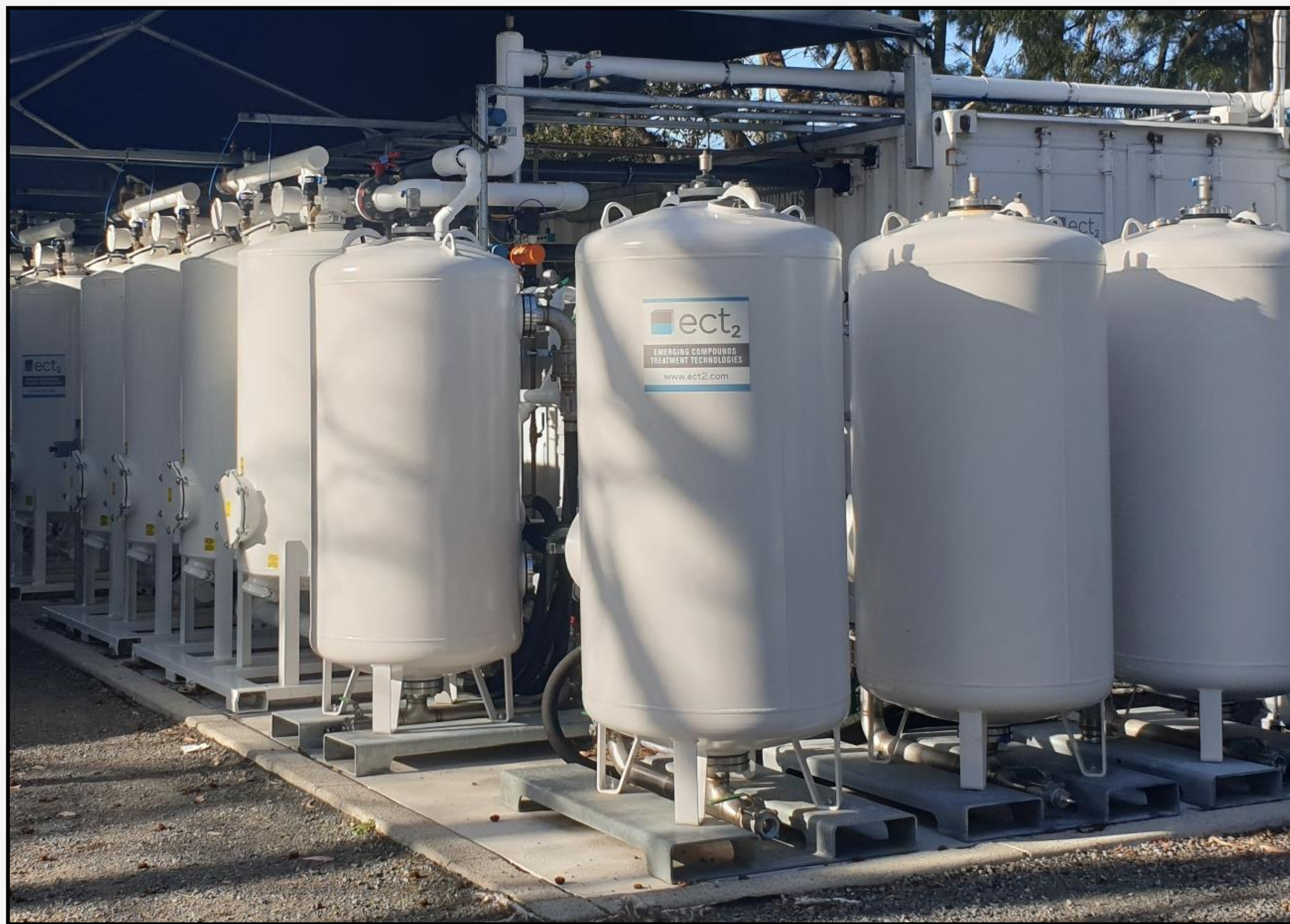
Moors Drain Water Treatment Plant
