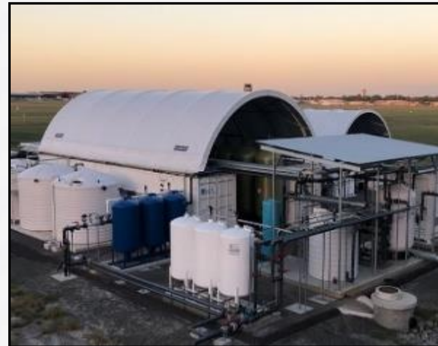
Western Region Water Treatment Plant
