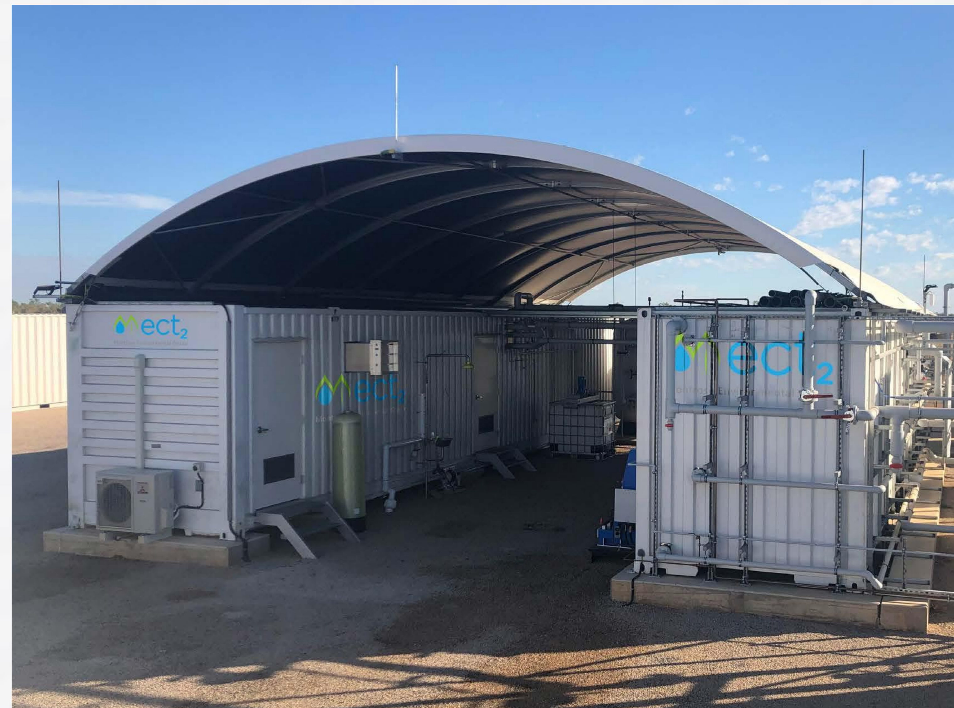
Groundwater treatment plant
