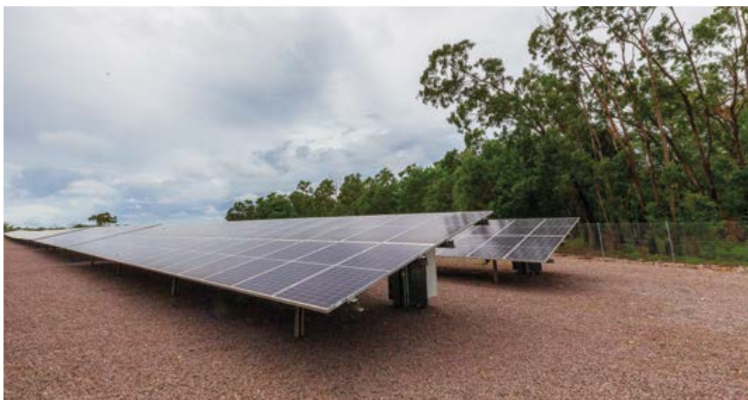
A new solar farm is installed at RAAF Base Darwin as part of the ADF's commitment to clean energy in the Northern Territory. IMAGE CREDIT: Corporal Madhur Chitnis.
