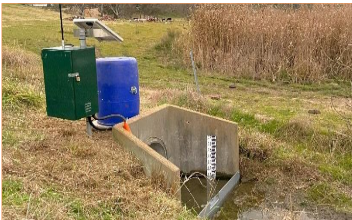
Surface water monitoring equipment installed in an on base drainage channel as part of the PFAS monitoring and assessment.
