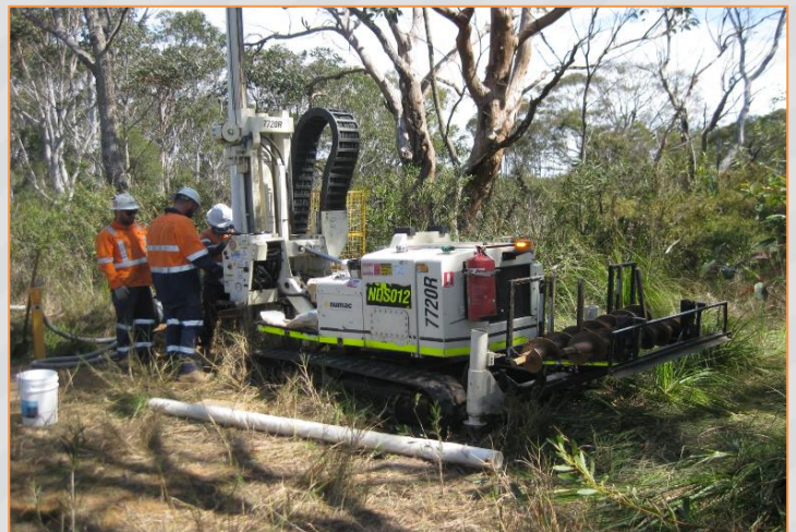
Image: Installation of an on-base groundwater extraction wellfield in the Western Region – September 2023.
