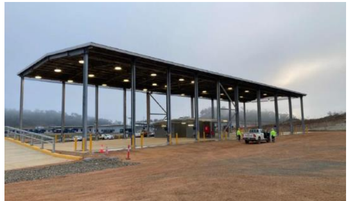
Above: Camp Logistics and Support – Mains power on
