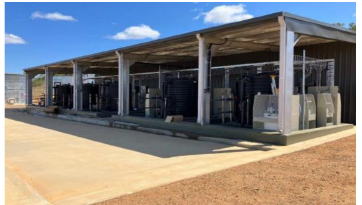
Above: Camp Tilpal Water Treatment Plant mechanical, electrical and piping works completed
