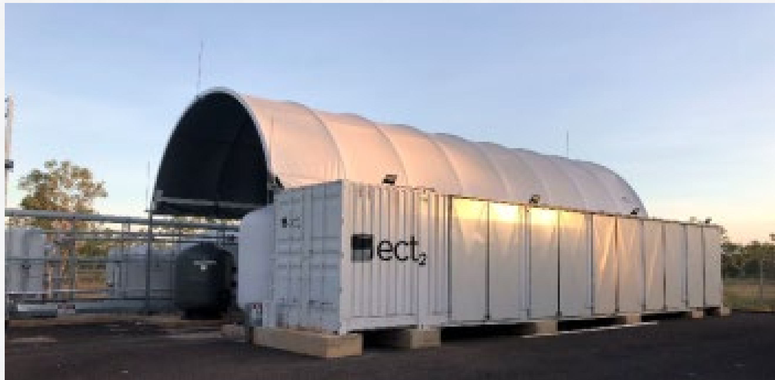
Fire Training Area Treatment Plant
