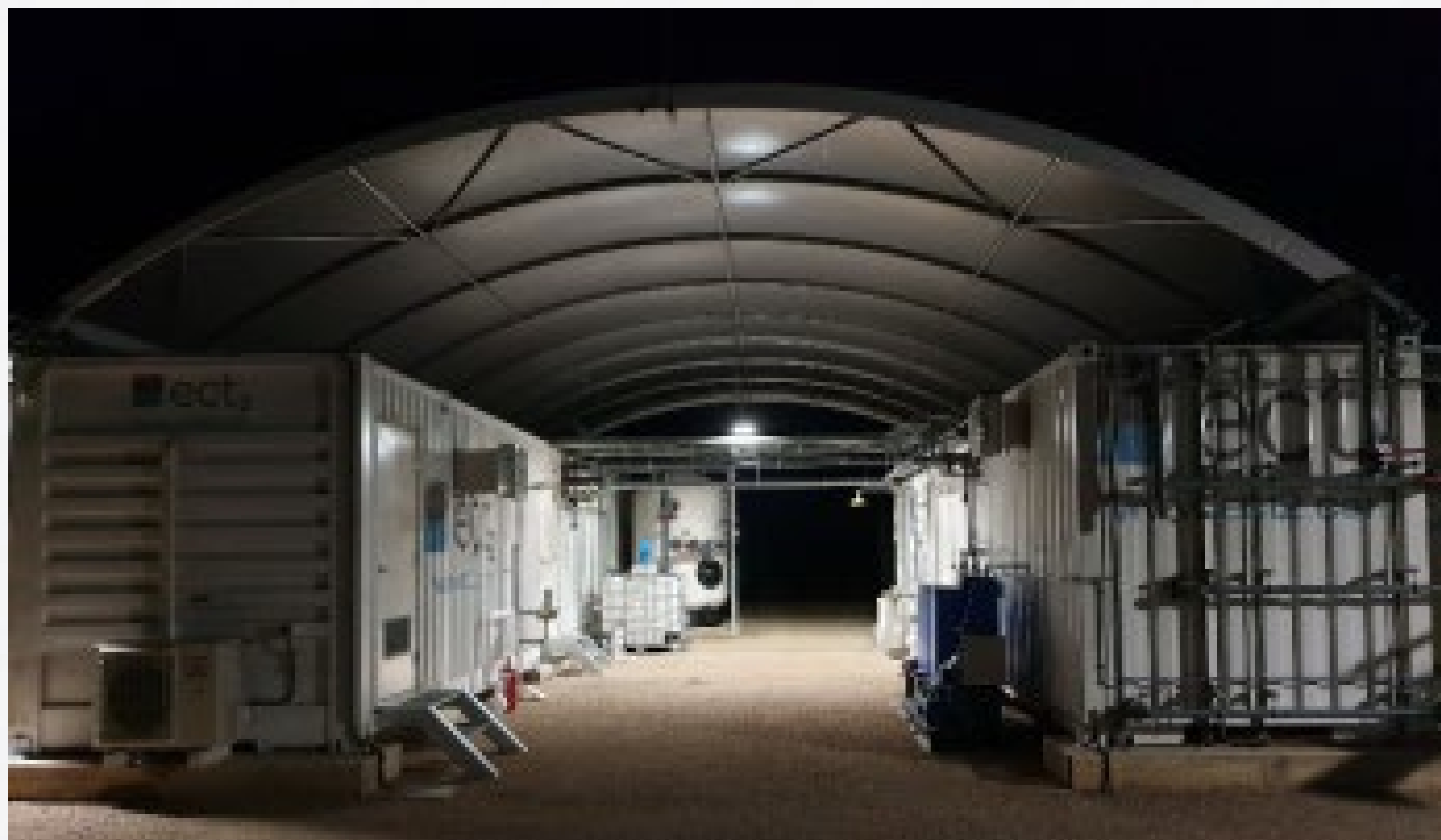
Fire Station Treatment Plant
