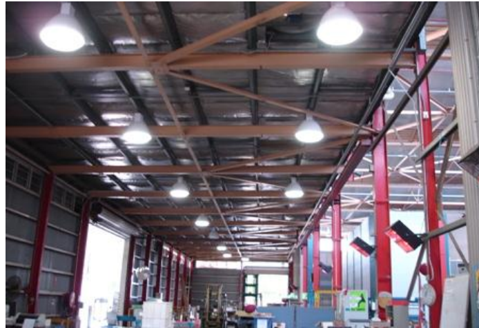
Natural lighting and high efficiency lighting, Warehouse, RAAF Base Amberley
