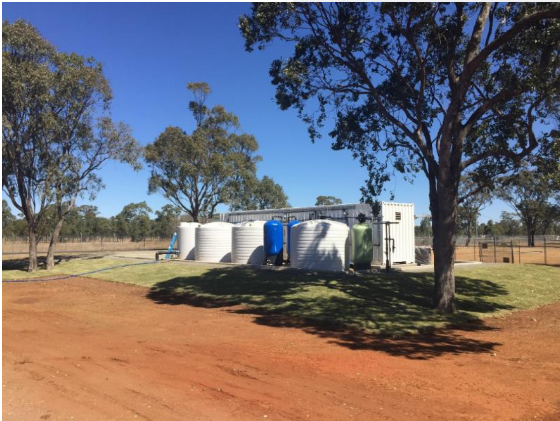
Above: Oakey Water treatment Plant
